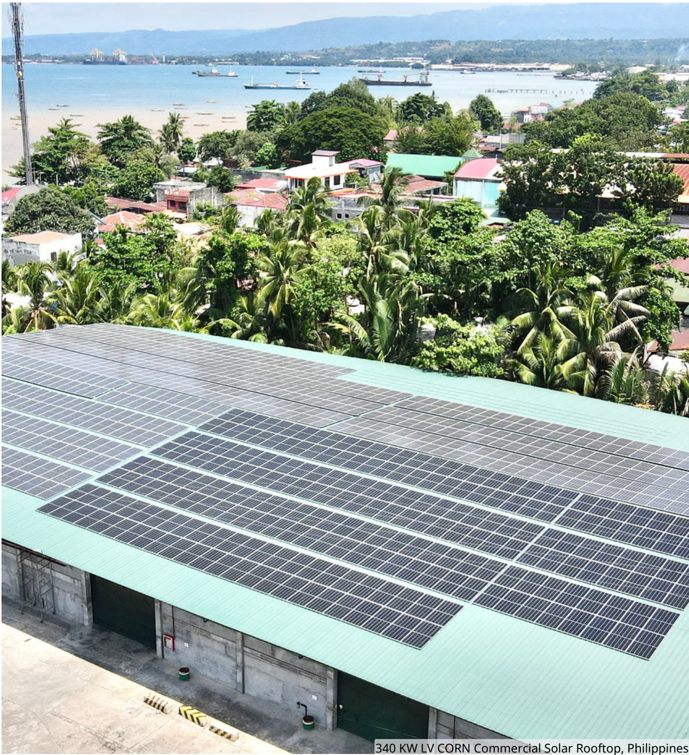
340 KW LV CORN Commercial Solar Rooftop, Philippines
